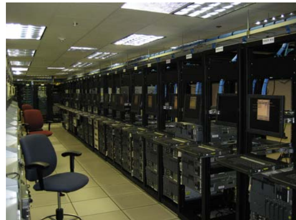
Servers on the Local Area Network at the Virginia Square Data Center.
