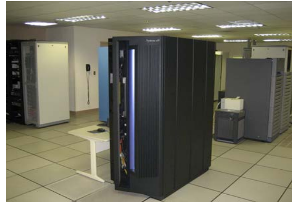
FDIC's mainframe computer at the Virginia Square Data Center.
